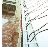
Snow Melting and De-icing
